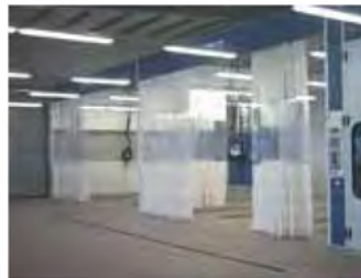
Down Draft Work Bays
